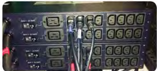
Red tape identifies the B side of the two cords supplying power to dual-corded devices. No tape is placed on the cord that is fed from the A side. In addition, blue tape is placed on each power feed to a single-corded device.
